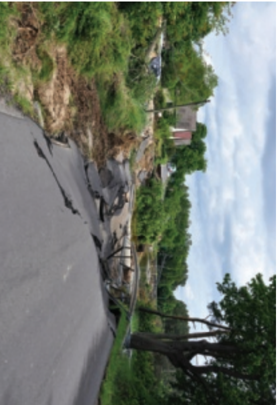
A road was washed out by floodwaters.
